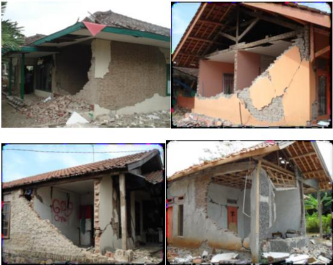
Fig 1: RC frame buildings with burnt clay bricks as infill walls are considerably vulnerable under seismic loadings
